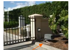
GATE OPENER. SOON TO BE REPLACED?
