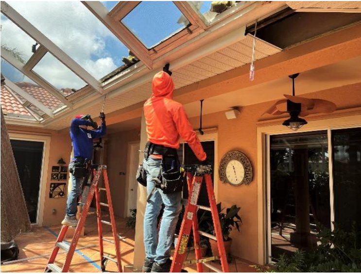
Replacement of fascia, soffits, downspouts and most gutters were included in the contract.
